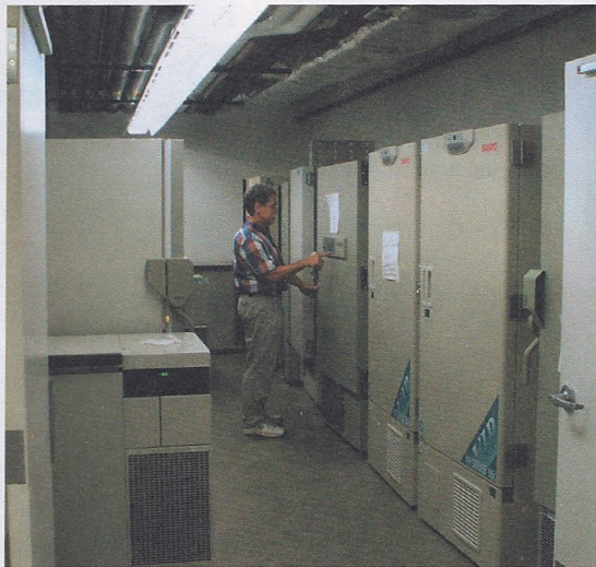
Fig. 6. A 650-ft 2 freezer farm provides an excellent service to investigators for the long-term storage of samples. All freezers in the farm are connected to an emergency generator.
